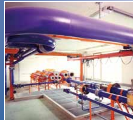
IMAGE OF TESTING HALL for control valve
