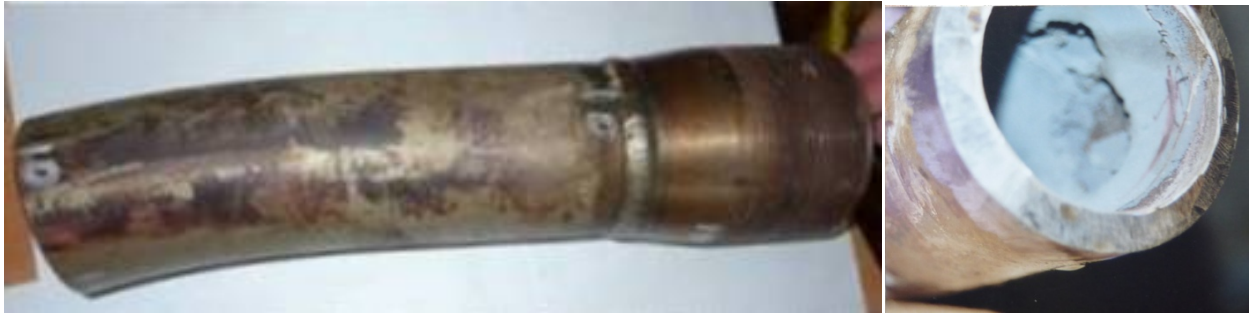
Picture 6a/b: The corroded 3" pipeline used for validation of the Digital Radiography Technique
