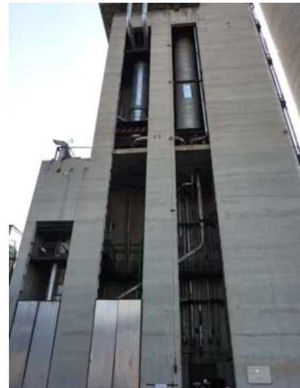
Picture 3: The civil structure of the high pressure synthesis section at Nitrogénművek Zrt. urea plant in Hungary
